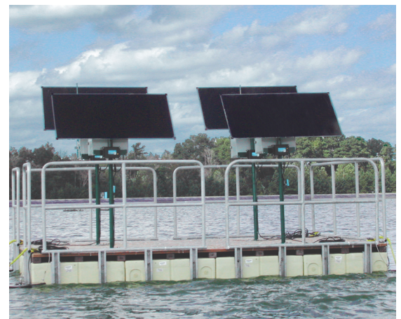
Four SonicSolutions ® solar panels on a float. Jacksonville, NC
